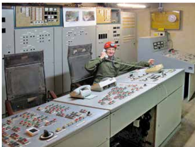
The Control Room: Tim Wellburn practises shutting down the bunker. Photo Clive Penfold
